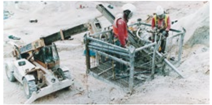
Installation of DYWI® Drill Hollow Bar Anchors at the Garden of Eden project in Great Britain
