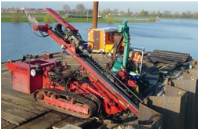
Hollow bar drilling from a floating barge for sheet pile tie back
