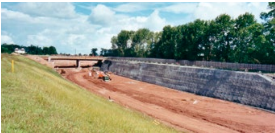
Steep cut slope with shotcrete facing for structural stiffness to resist bulging
