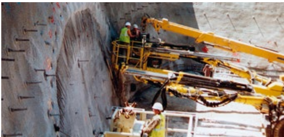
Self-drilled hollow bars for the stabilization of a tunnel portal and approach cutting
