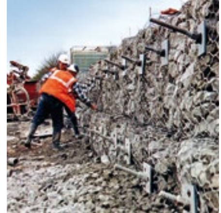
Soil nailed gabions at the toe of a slope
