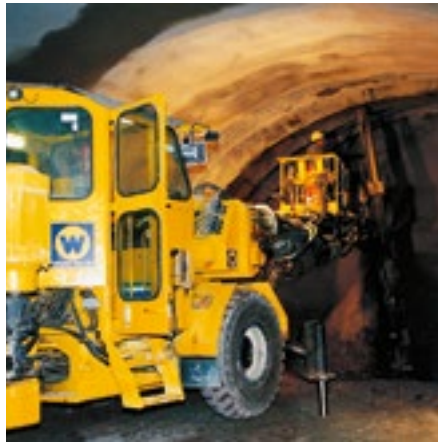
Stabilization of a tunnel portal using DYWI® Drill Hollow Bar Anchors, Ø32mm – Thuringia, Germany
